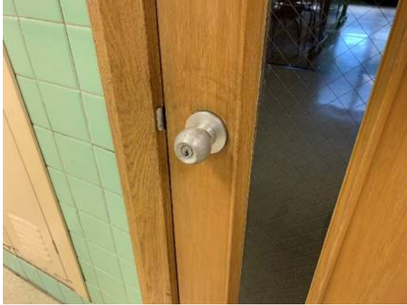
Photo A08 – Non-compliant Door Handle
