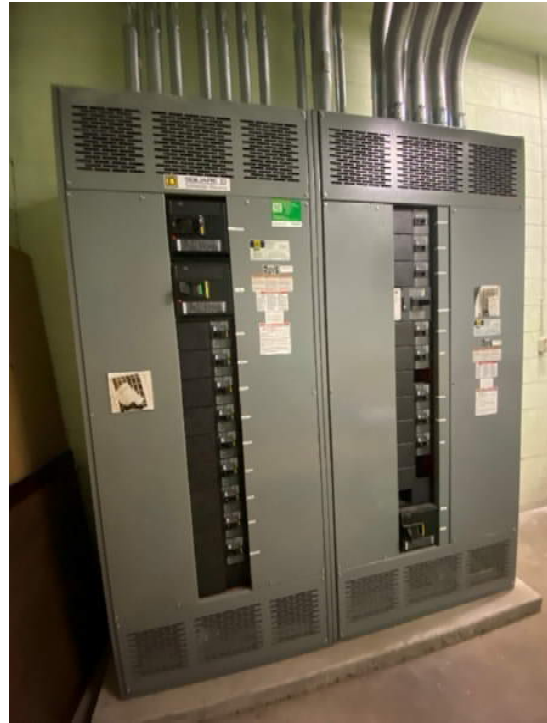
Photo E02 – Main Distribution Panel
