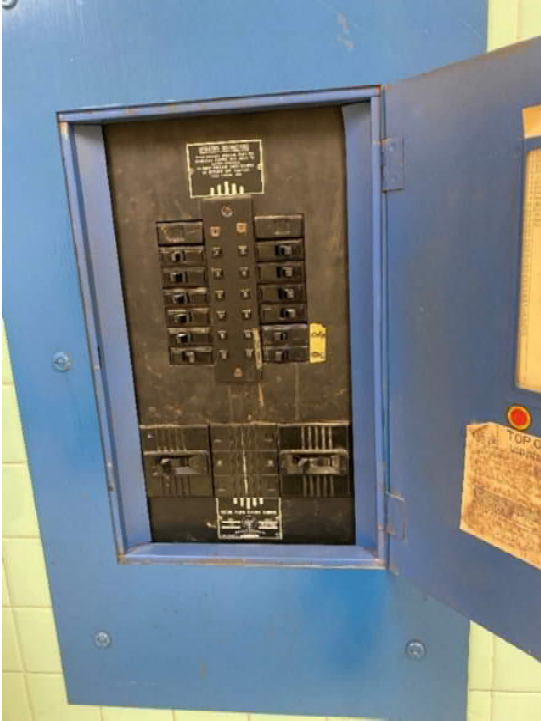
Photo E03 – Branch Circuit Boards
