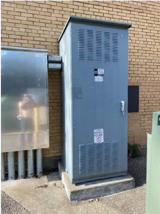
Photo E01 – Service Entry Switch
