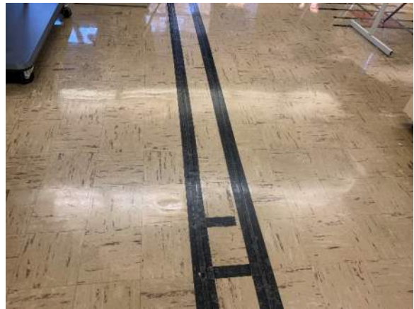
Photo A19 – Asbestos Floor Tile
