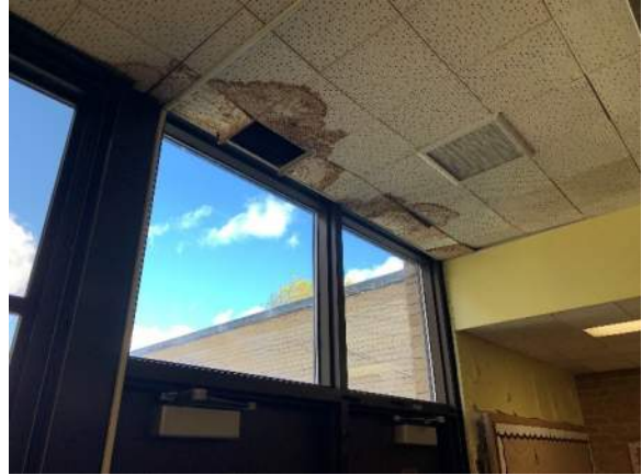
Photo A09 – Water Intrusion Damage
